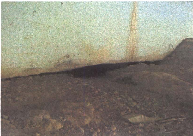
SETTLEMENT AT ABUTMENT #1 EITH EXPOSED PILE
